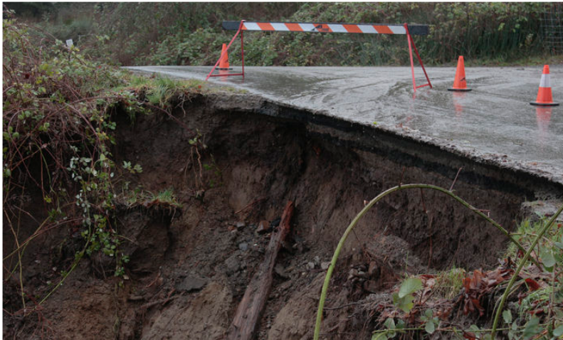
Eroded roadside in the 700 block of Walker's Hook Road on Monday. Marc Kitteringham / GI Driftwood
