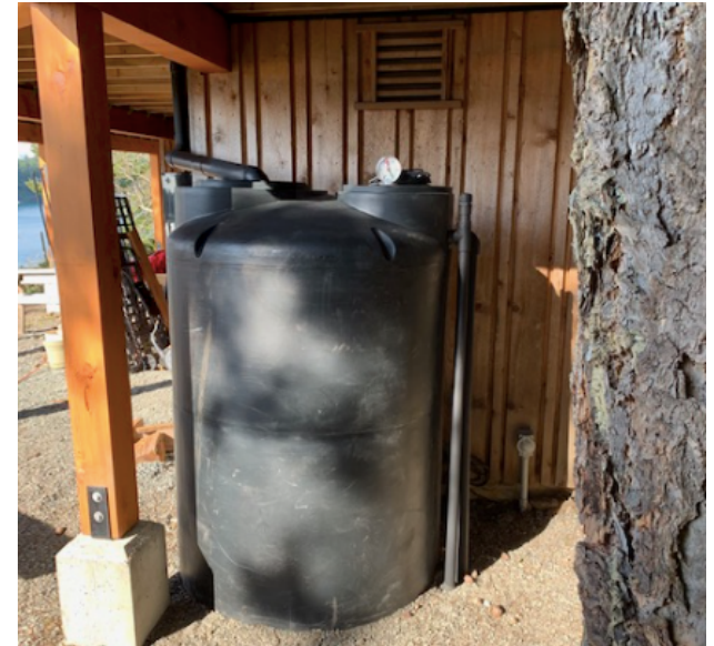
PUMP TANK NEXT TO HOUSE PUMPS RAIN TO STORAGE TANKS A FURTHER DISTANCE AWAY.
