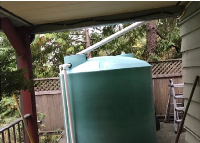
GRAVITY-FED DRY TRANSPORT SYSTEM TO 1,000 USG TANK.
