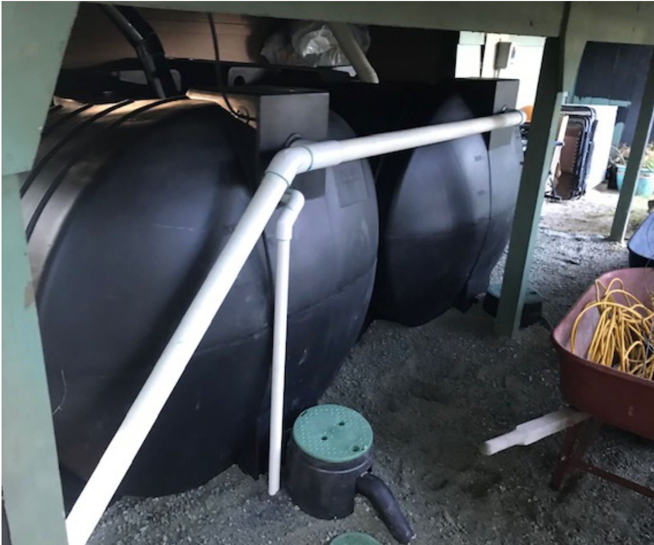
TWO 7,550L (2,000 USG) POLYETHYLENE TANKS WITH INTERCONNECTING PIPING AND PROTECTIVE VALVE BOXES (BEFORE FINAL BACKFILL). COLLECTION FROM PUMPHOUSE ROOF.
