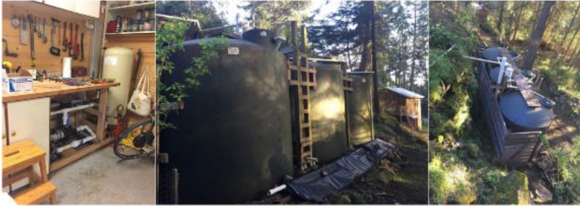
Figure D7. Case study S1 images taken by Kendra Anderson during site visits to gather further details on RWH systems that exist on SSI. A UV filter is used to bring water up to potable quality, and a pump transports water from the three large 3,000 gallon tanks to the house for use.
