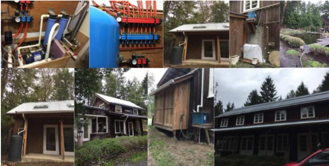
Figure D1. Case study B1 images taken by Kendra Anderson during site visit on April 22, 2017 to gather further details on RWH systems that exist on SSI. Collection of rainwater occurred off all roofs on the property, which are linked and controlled via piping and valves.
