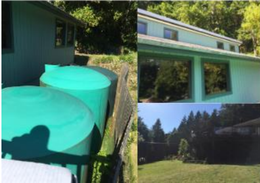
Figure D5. Case study C2 images taken by Kendra Anderson during site visit May 29, 2017 to gather further details on RWH systems that exist on SSI. Water is collected off the workshop roof and held in three cisterns with a combined volume of 6,600 gallons, used to water the garden area.
